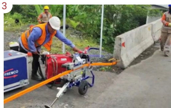
DuctRod RAPID in use pushing the micro duct into the concrete barrier a distance of 280m/306yds
